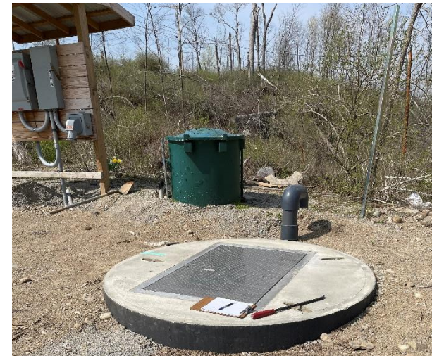
Murwood Lift Station
