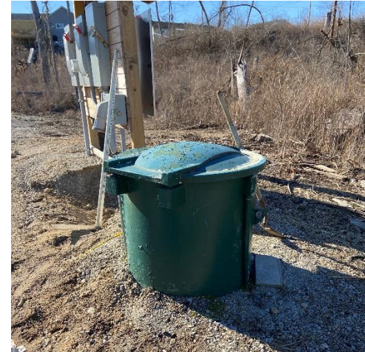
Murwood Lift Station
