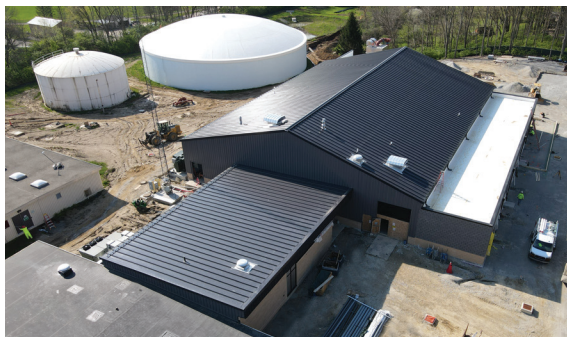
Construction at the Northwest Regional Water Treatment Plant nears completion, allowing GCSED to expand system capacity and improve system reliability.
