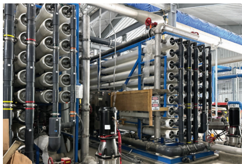
New reverse osmosis treatment system at the water treatment plant will deliver softer water and improve water quality.
